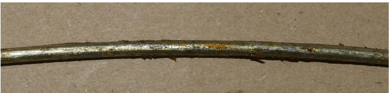
Figure 3 Condition of core steel strand – Tag ID 271
