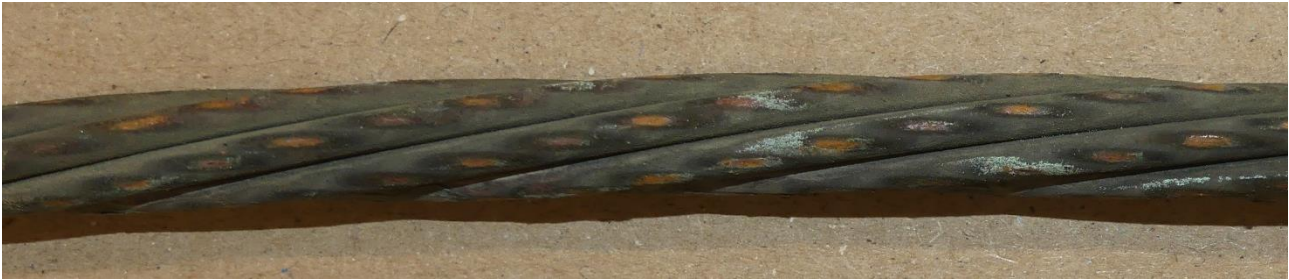
Figure 6 Outer surface of inner copper strands – Tag ID 140
