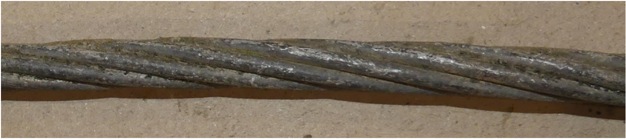
Figure 9 External surface of the conductor – Tag ID 005
