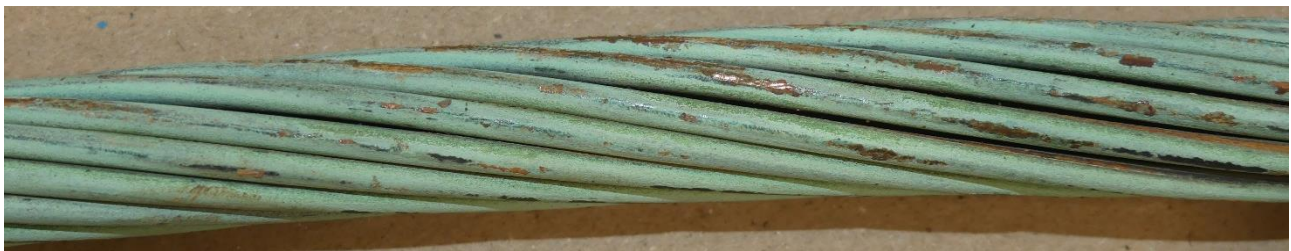
Figure 4 External surface of the conductor – Tag ID 140
