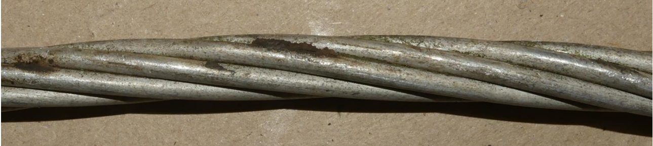
Figure 1 External surface of the conductor – Tag ID 271
