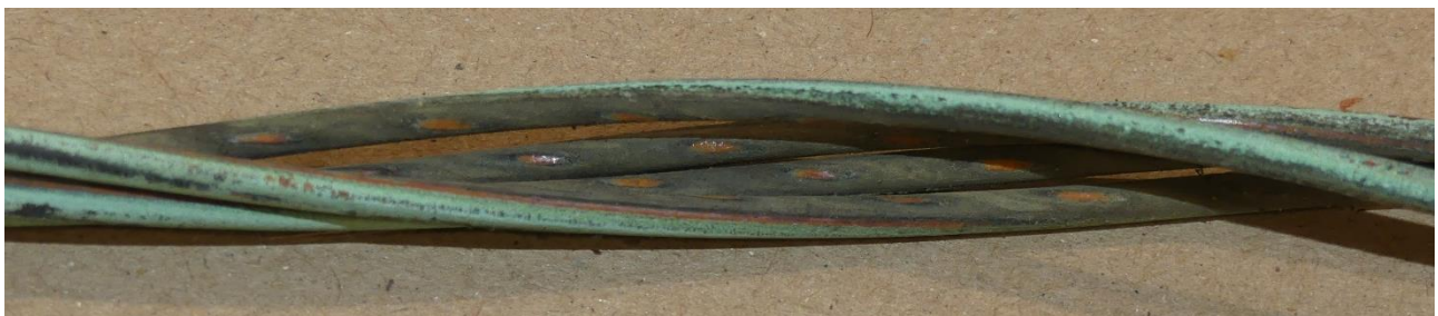
Figure 5 Inner surface of copper strands – Tag ID 140
