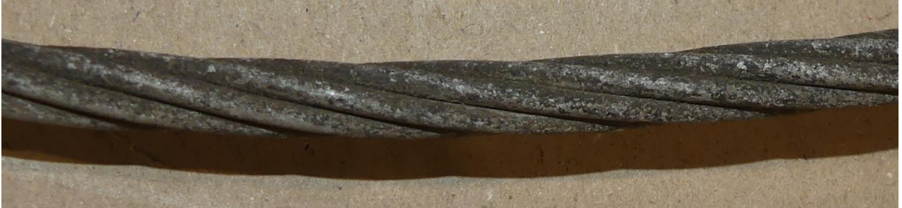
Figure 12 External surface of the conductor – Tag ID 001
