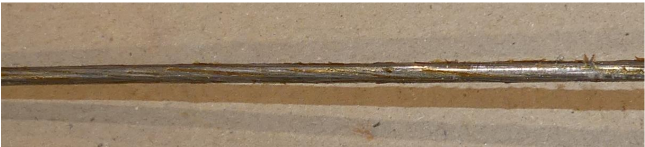
Figure 11 Condition of core aluminium strand – Tag ID 005
