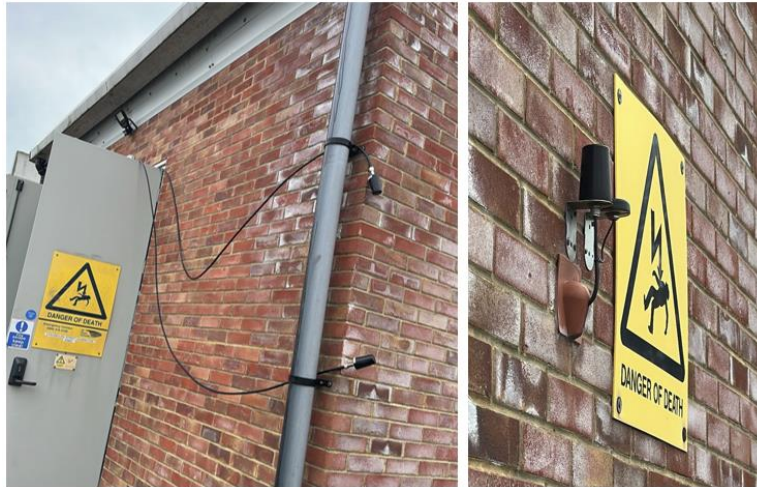
Figure 2-10 – The left-hand side shows the temporary test setup with external antennas, while the right-hand side illustrates a potential permanent installation.
