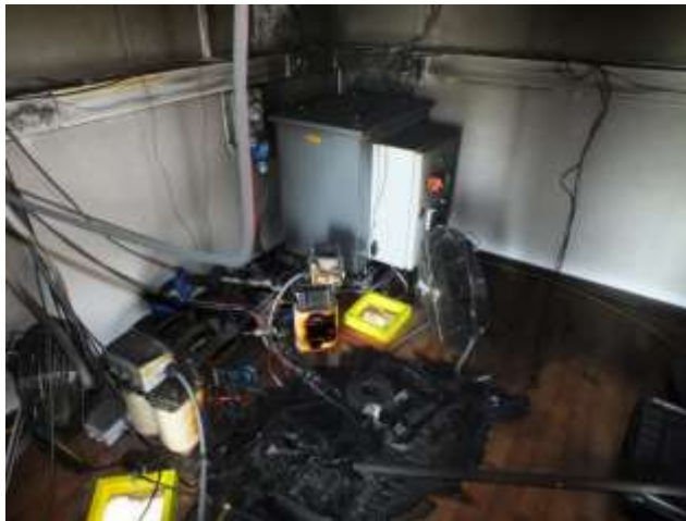
Figure 8 Power Factor Correction Unit
