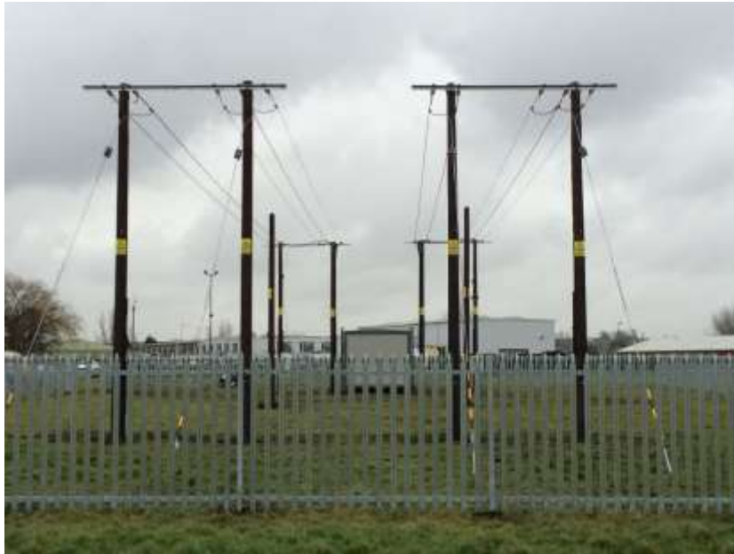
Figure 3 OHL conductor configurations at Terminal H-poles
