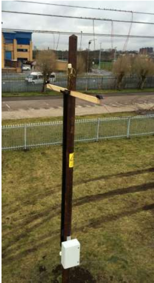
Figure 5 Weather monitoring equipment installed on freestanding intermediate wood poles and conductor thermocouples
