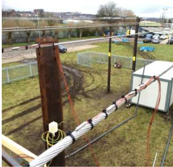
Figure 4 Example of Conductor Thermocouple installation
