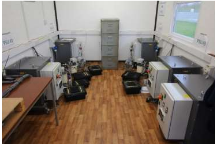
Figure 6 Portacabin (Hut) Interior – operational equipment
