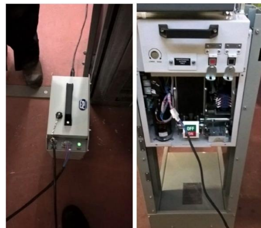
Figure 3: Portable power pack (left) plugged into retrofit VOR-M CB (right) during testing of the power pack
