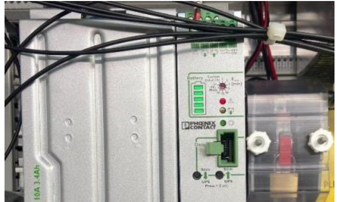
Figure 22: UPS Fault Alarm Indication in Phase L2
