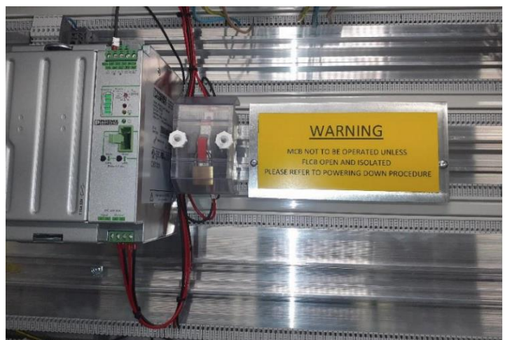
Figure 21: Control System Power Supply MCB Locked in the 'On' Position, with Cover and Labelling Applied
