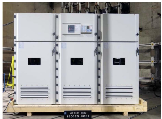
Figure 19: FLCB panels after short time current withstand testing
