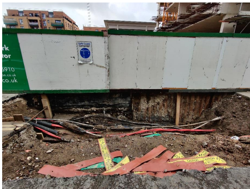
Figure 12 Large sinkhole that has developed adjacent to construction site, blocking one half of the road
