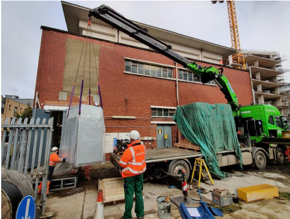
Figure 6 Delivery of FLCB to the network demonstration site
