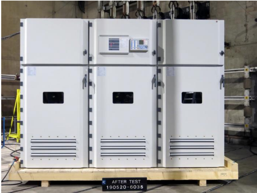
Figure 2 FLCB panels after short time current withstand testing
