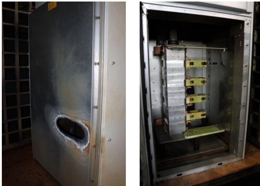
Figure 3 Rear of FLCB panel (left) and front of panel (right) after failed internal arc test
