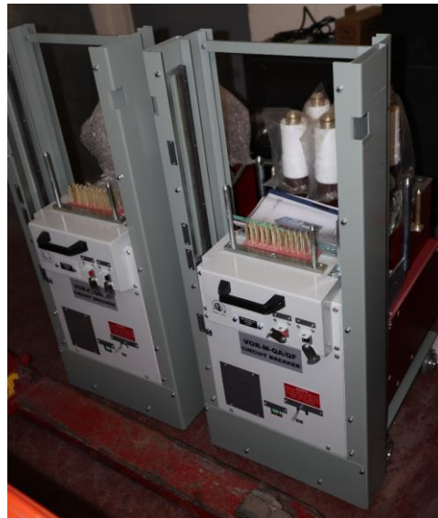
Figure 9 Retrofit circuit breakers prior to being installed into busbar extension
