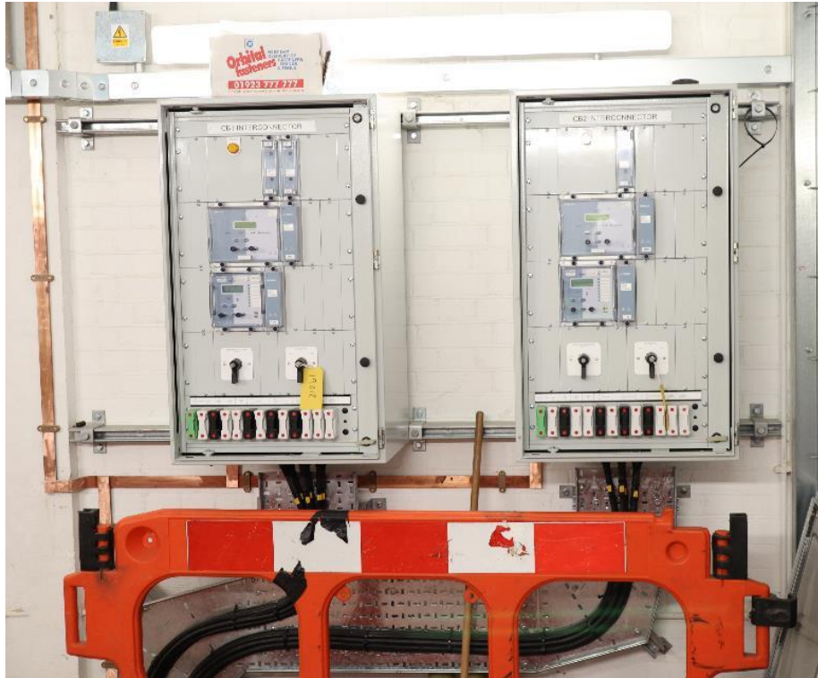
Figure 5 Protection panels installed at network demonstration site
