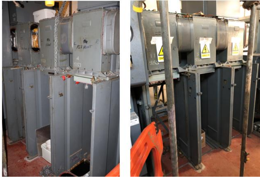
Figure 8 Progress of busbar extension with retrofit circuit breakers to still be added
