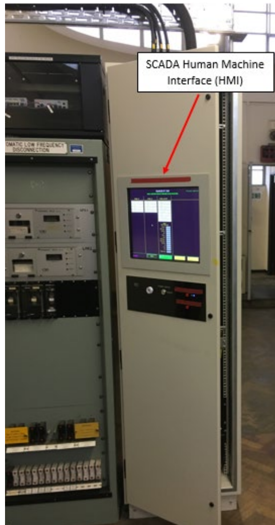
Figure 2 SCADA panel with HMI screen which shows alarms from the FLCB and other protection equipment
