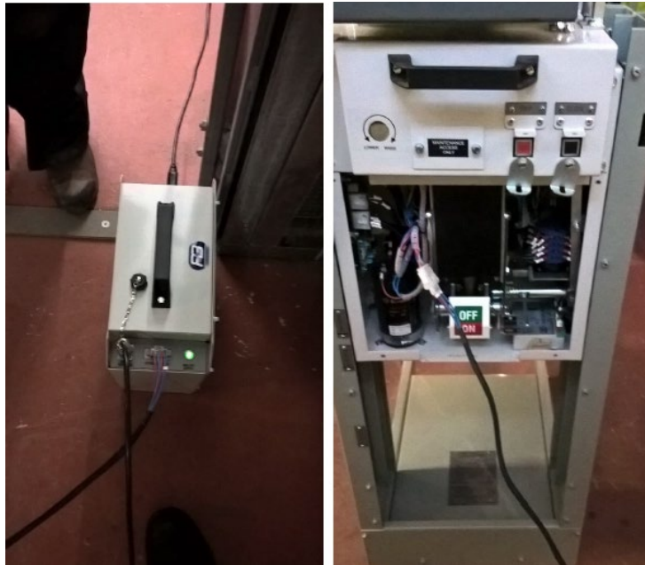
Figure 7 Portable power pack (left) plugged into retrofit VOR-M CB (right) during testing of the power pack
