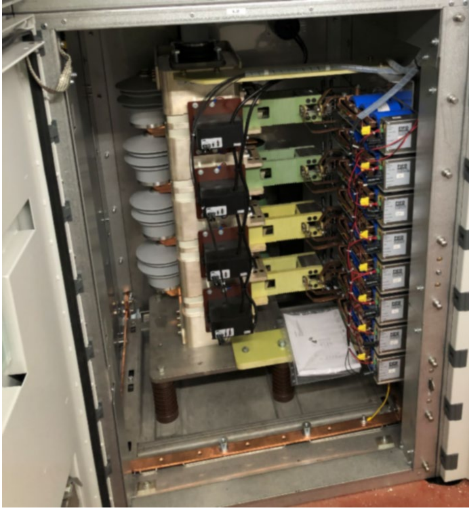
Figure 3 HV compartment of the FLCB
