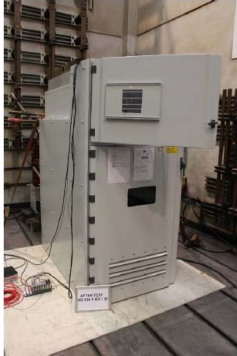
Figure 37 – FLCB after final interruption test
