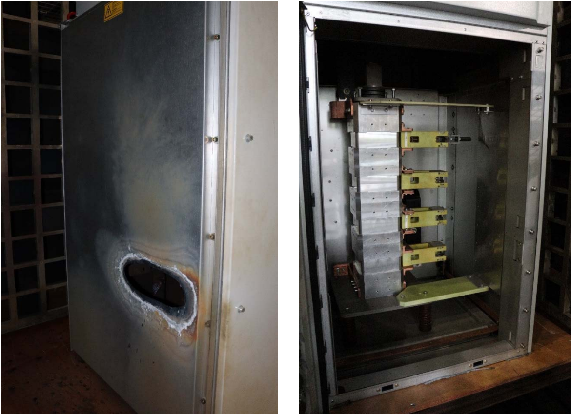
Figure 27 – Rear of FLCB panel (left) and front of panel (right) after failed internal arc test
