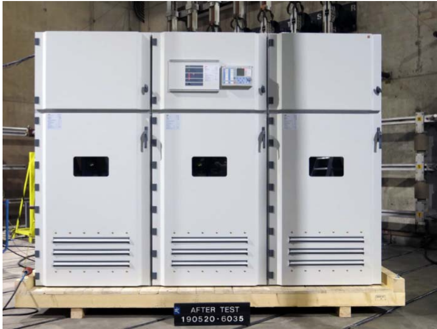
Figure 49 – FCLB panels after short time current withstand testing
