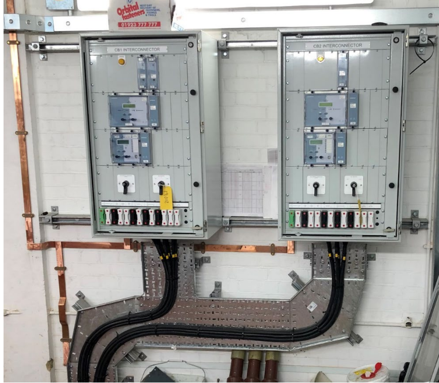
Figure 21 Protection panels house differential protection relays and overcurrent protection relays for the two adjacent circuit breakers CB21 and CB22
