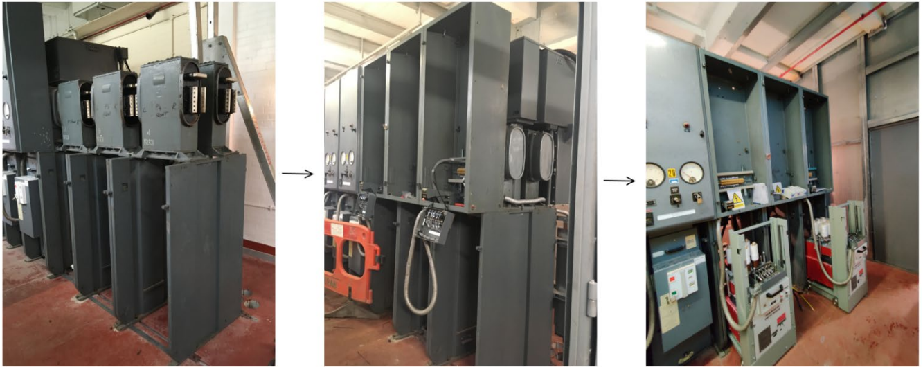
Figure 17 Sequence of work to extend the existing busbar – spare bays in place (left and middle) and retrofit circuit breakers ready to be put in position (right)
