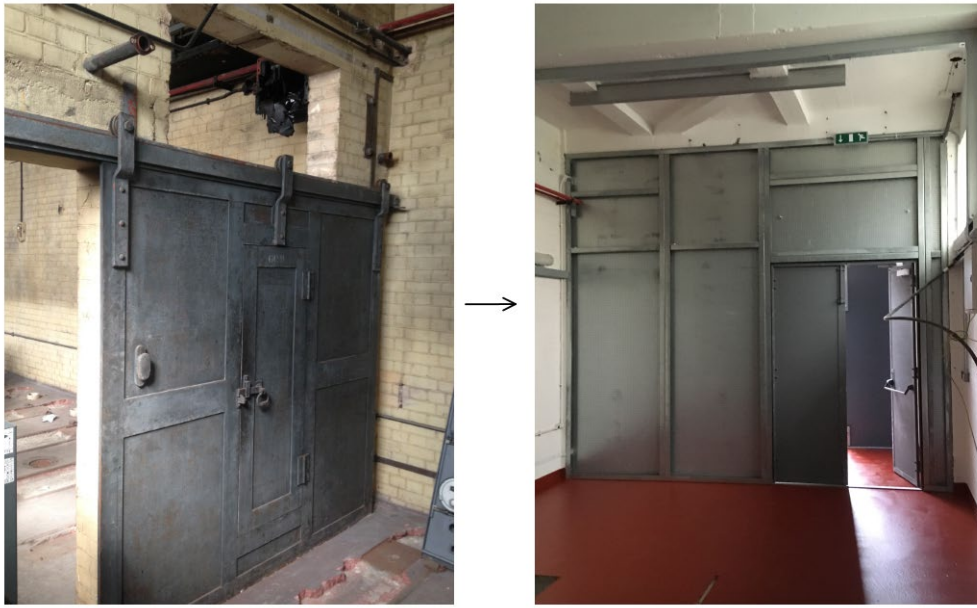
Figure 12 Second internal wall requiring replacement (left) and newly installed durasteel wall and door (right)
