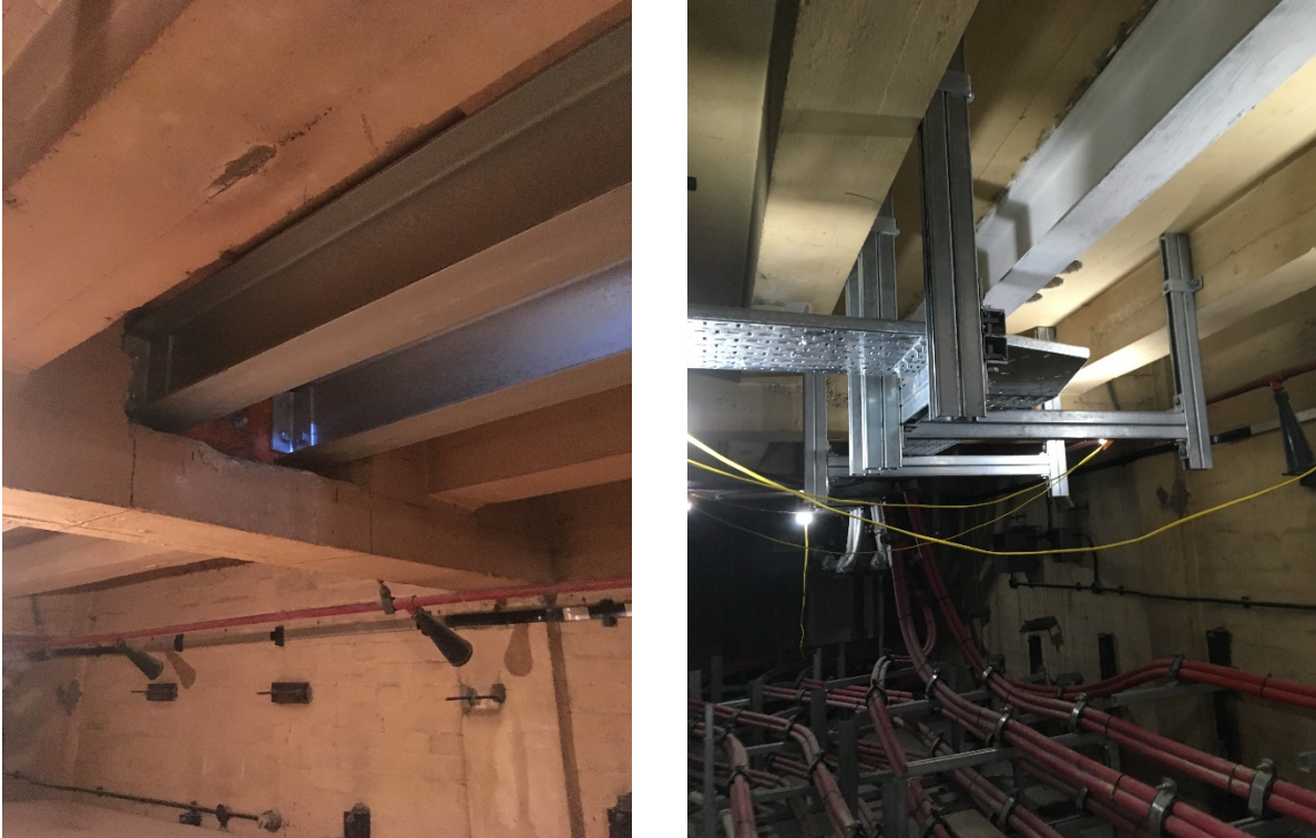
Figure 14 Supporting steelwork in the basement (left) and cable trays added for multicore cables (right)
