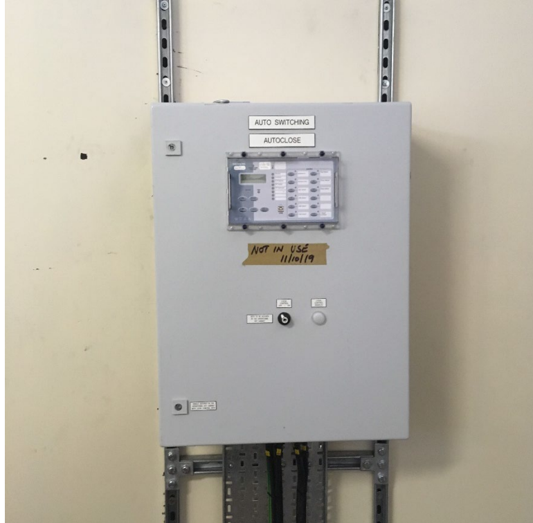
Figure 26 Auto-close panel installed
