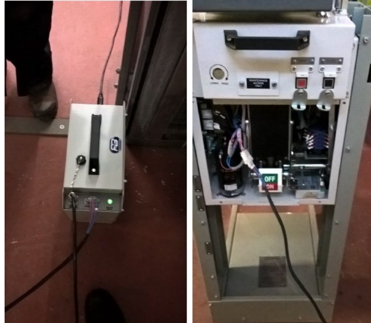
Figure 43 Portable power pack (left) plugged into retrofit VOR-M CB (right) during testing of the power pack
