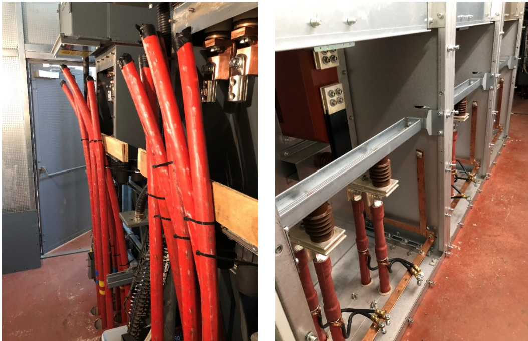
Figure 18 HV cables ready to be terminated to the existing switchgear (left) and completed HV terminations to the FLCB (right)
