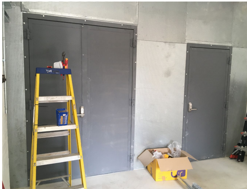
Figure 11 Newly installed durasteel wall and doors to allow for extension of the existing busbar
