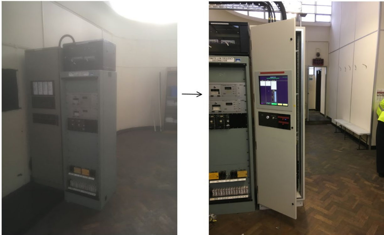
Figure 22 Existing SCADA equipment (left) and additional SCADA panel added (right) which includes Human Machine Interface (HMI)
