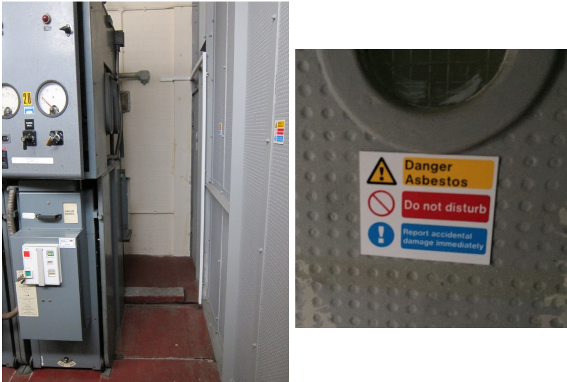
Figure 10 Existing fire protection wall requiring relocation for busbar extension which was replaced due to containing asbestos
