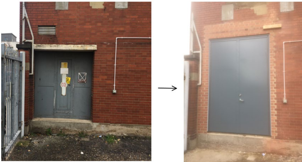
Figure 13 Existing door (left) replaced by larger door (right) to provide access for the FLCB
