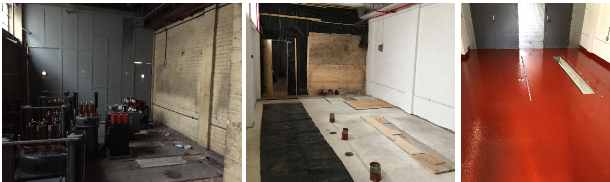
Figure 9 General sequence of works to ready the room for FLCB installation. Before works (left), screed poured and levelled, walls painted and holes drilled (middle) and finished floor (right)
