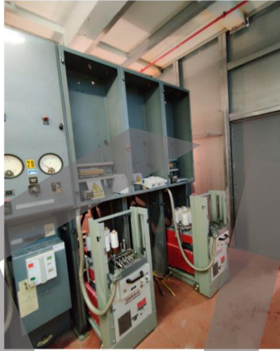
Retrofit vacuum circuit breakers installed
