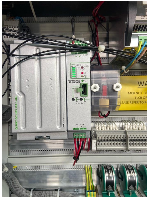
Figure 7 UPS fault alarm indication in phase L2
