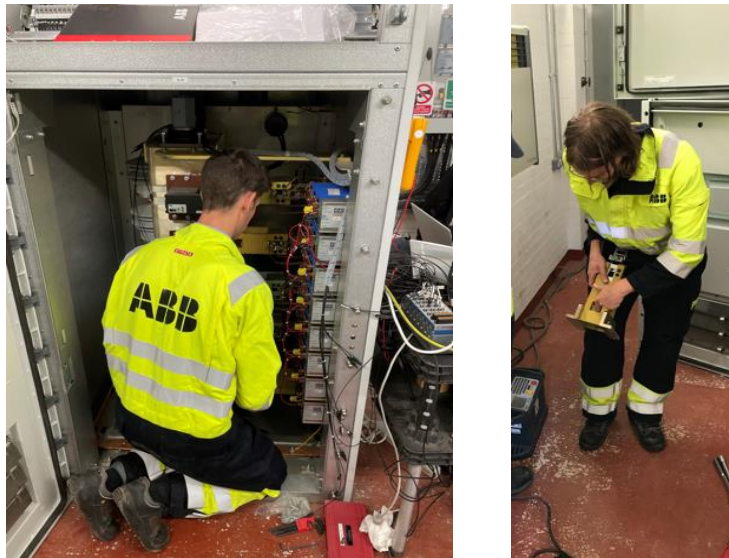
Figure 3: ABB Engineers carrying out the site inspection and maintenance. The picture on the right shows the mechanical switch that was replaced.
