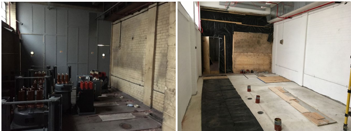
Figure 6 Existing room prior to site works commencing (left) and progress of completing site works (right)
