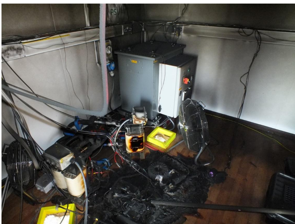
Figure 2 Fire damaged Power Factor Correction Unit 7 th June 2016
