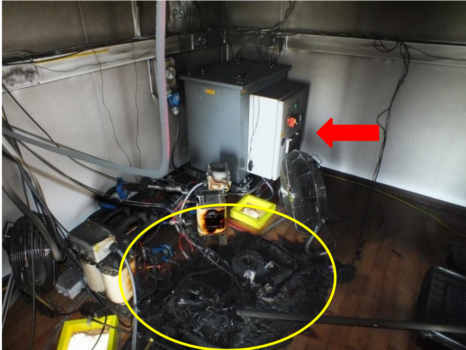
Figure 1 Location of fire within porta-cabin. Power supply unit (PSU) 4 indicated by red arrow.
